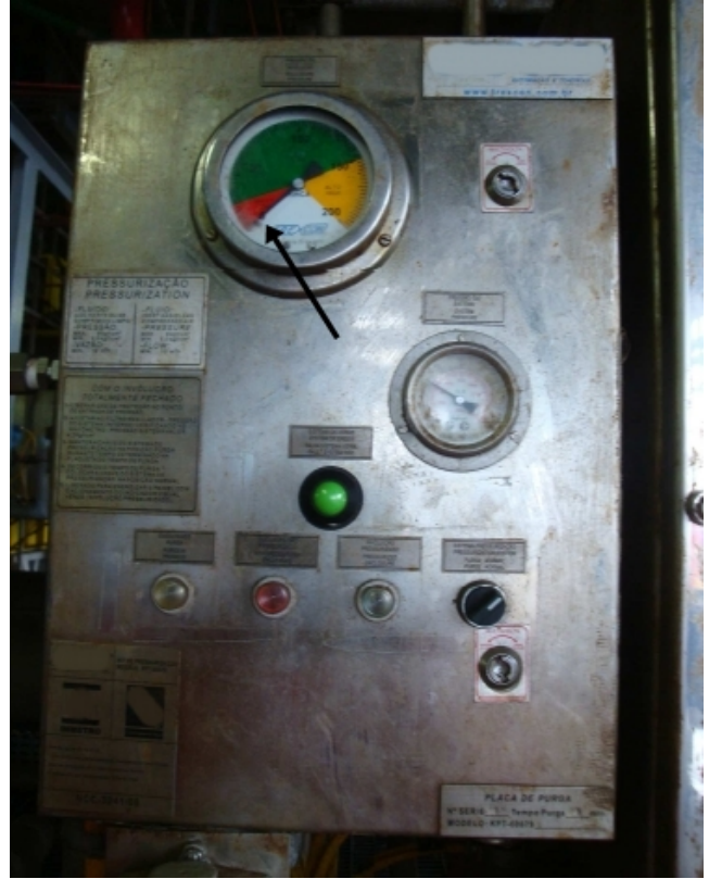
Fig. 10 Underpressure indication in an Ex-p enclosure
