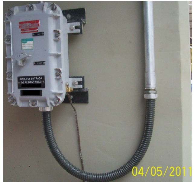
Fig. 11 A plastic flexible conduit connected to an Ex-d enclosure without a conduit sealing device.
