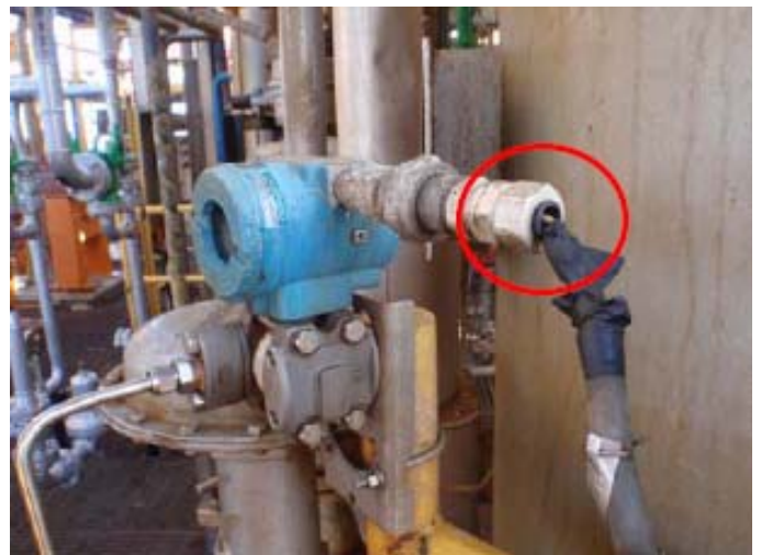
Fig. 7 Cable gland incorrectly "filled" with electrical insulating tape.
