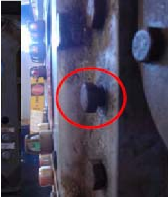
Fig. 4 Loose screws of an Ex d enclosure.
