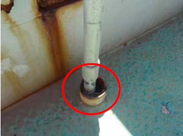
Fig. 8 Floor penetration without a sealing compound.
