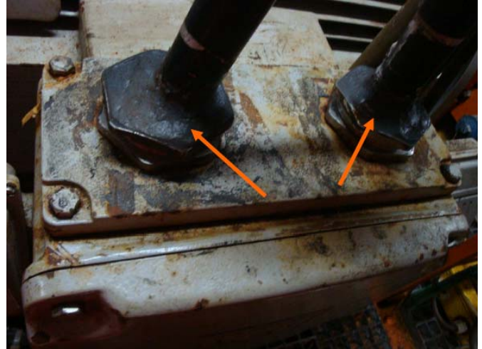
Fig. 6 Cable-glands incorrectly "filled" with silicone sealant on an Ex e enclosure.
