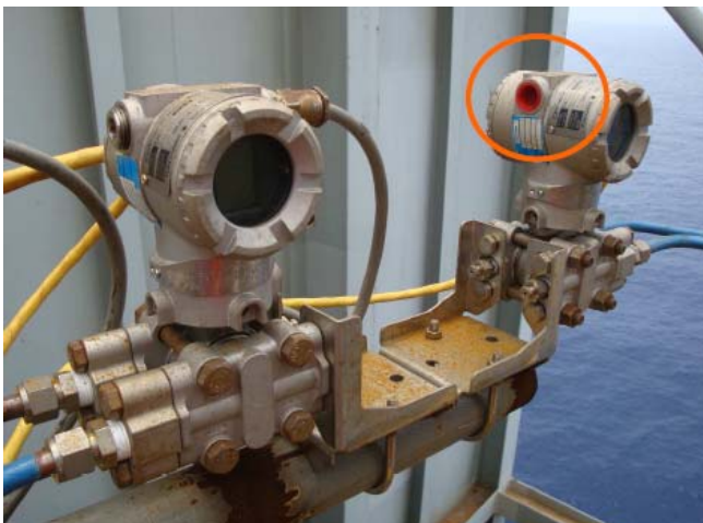
Fig. 1 Unsuitable plastic blanking element in an Ex d enclosure.
