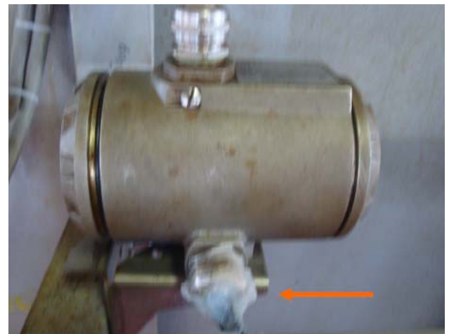
Fig. 3 An unused cable entry of an Ex d instrument was closed with a room temperature vulcanized (RTV) silicone sealant instead of a certified metal close-up plug.
