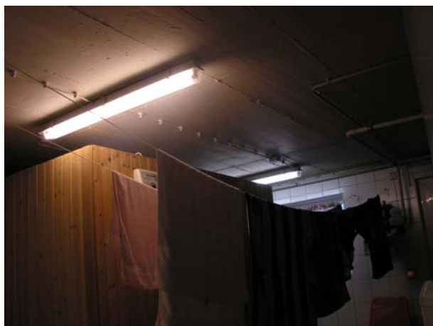
Fig. 3.15: Fluorescent lamps in a residential washroom with magnetic ballasts and electronic starters: Only one lamp replacement within well over 30 years
